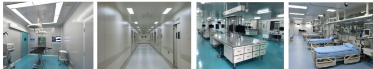
洁净手术室 Clean Operating Room
